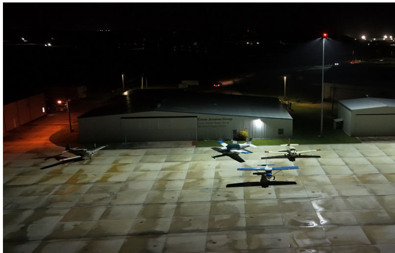
Newly installed high mast lighting
